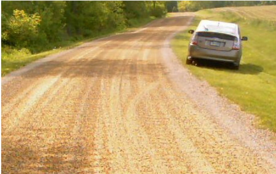
Figure 4. Ruts in a gravel road.
